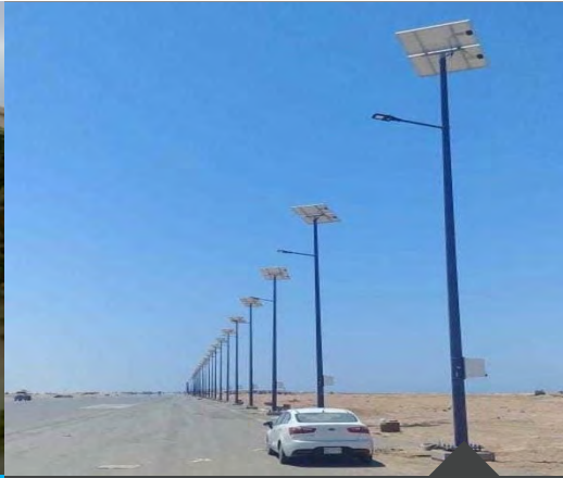
NEOM MAIN STREET LIGHT PROJECT
